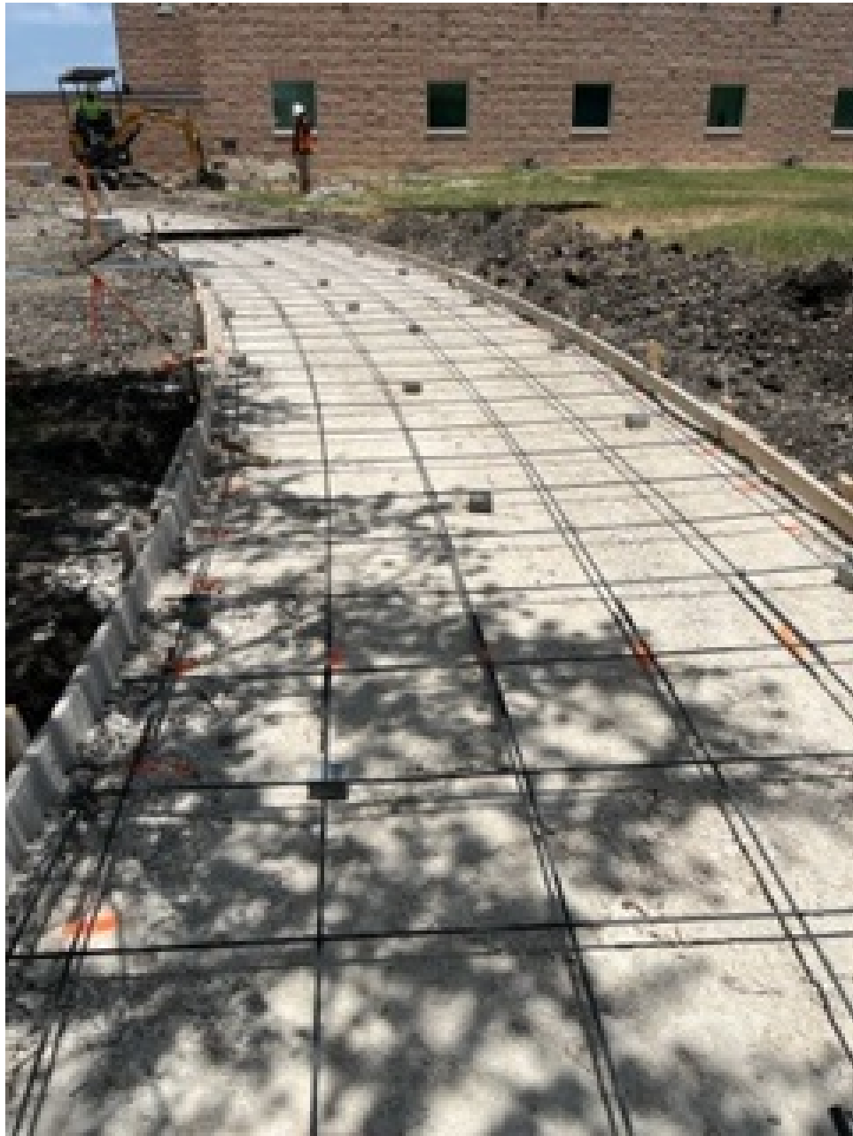
East sidewalk with flex base and rebar. Pouring concrete for a portion of it.
