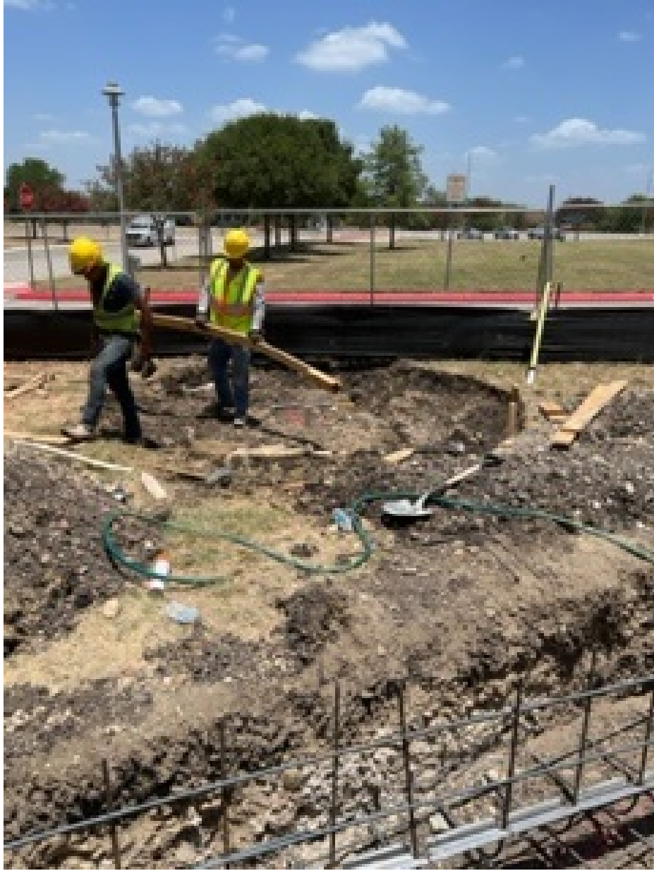
Workers preparing one of the sites for a proposed concrete pad. 6" of flex base and rebar will be installed for the upcoming pour. Concrete depth will be of 5".
