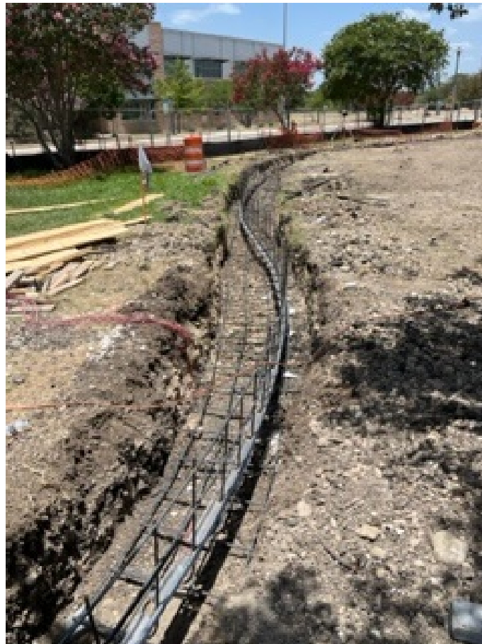
Digging a trench for the proposed low landscape wall. The trench prepared with rebar to pour concrete for its base.
